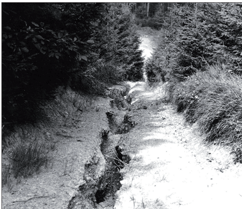
Phot. 6. Forest road damaged by water (phot. by L. Buzek)
